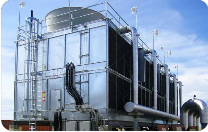
Figure 1: Improving cooling tower efficiency can unlock production gains
